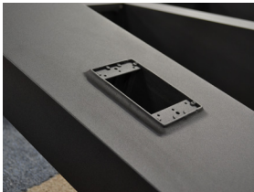
GFCI GFCI Box
